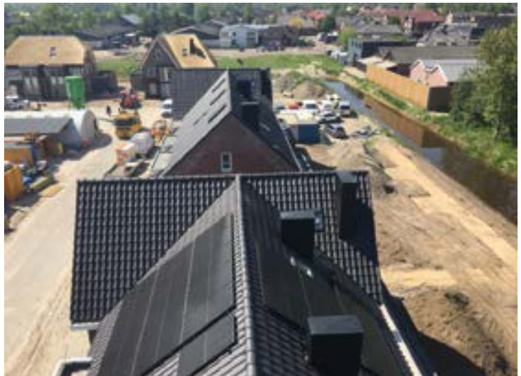
Combined with solar panels.
